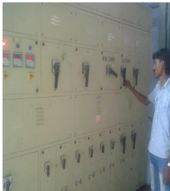
Switching on the main power panel
